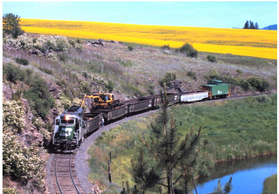
A 1994 Burlington Northern work project left a large number of tie ends and other scrap alongside the WI&M right-of-way. To clean up, BN dispatched this train of gondolas and a small crane with a claw on its arm to pick up the scrap material and place it in the gondolas. When Carl Sonner took this image, the crew had just realized that the crane would no longer rotate, and the arm would impact the rock walls if the train continued forward. Instead, they had to back the train to Princeton and repair the crane while allowing the eastbound freight train to pass.
