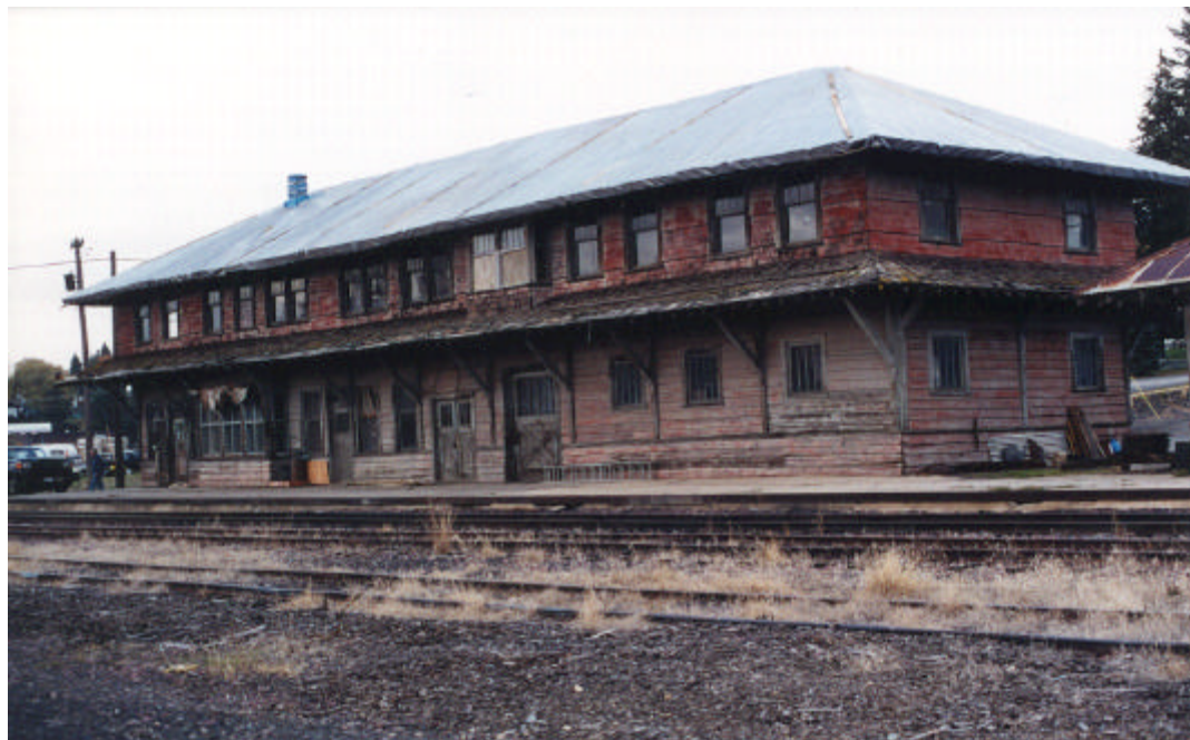
The Potlatch depot shows off its new, albeit temporary, roof and blue tarped chimney. The PRCC high-rail truck shows up on the platform just as the last of the Clearwater Power boom and bucket trucks head for the barn in Princeton. In spite of the gloomy day, the winds were light and no rain fell. The donated hay tarps secured onto the roof will protect the second-floor plaster/lath walls and the wooden staircase from further damage this winter. HPG photograph
